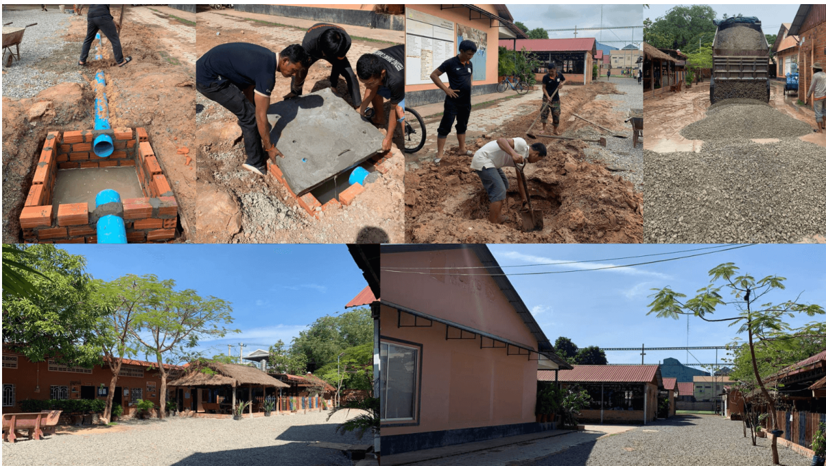
New FDC Drainage System
